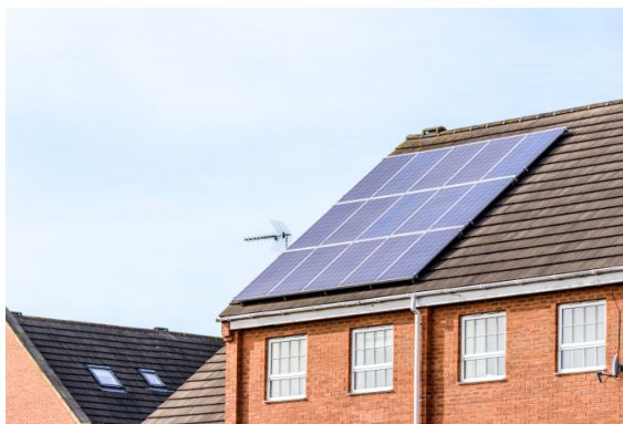
Photovoltaic panels generating electricity. Alternatively solar thermal roof panels can be used to generate hot water.
