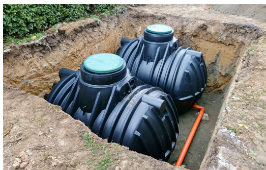
An example of a rainwater harvesting tank
