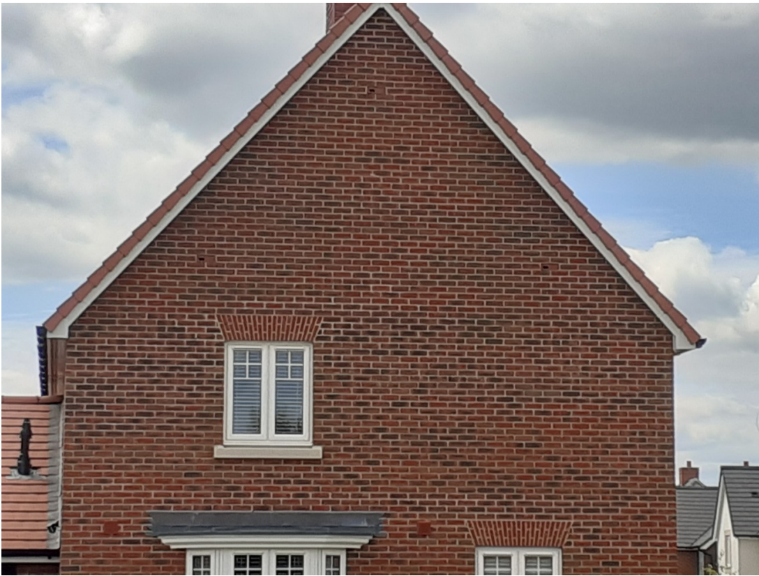
Bat and bird bricks on the gable end of new houses in Buckinghamshire Source: Herts and Middlesex Wildlife Trust
